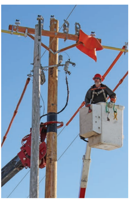
Lead Lineman Rick Bowers (left) replaces a utility pole with the help of Apprentice Lineman Zach Hart (opposite page), who operates equipment to hold the new pole in place. Bowers, Hart, and Lead Lineman Phil Pickering (cover) are just one of several co-op and contractor crews completing Firelands' current work plan.
